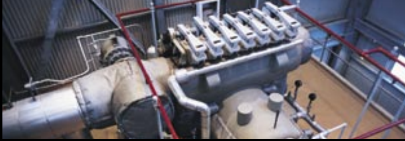
This 15 MW topping steam turbine reduces steam pressure from 400 psig (29 bar) to 100 psig (8 bar) and generates electricity for a rubber polymer manufacturing facility.
