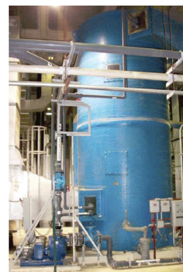
PRD Tech's Biofilters at Sanitation District No. 1 Plant, Florence, KY
